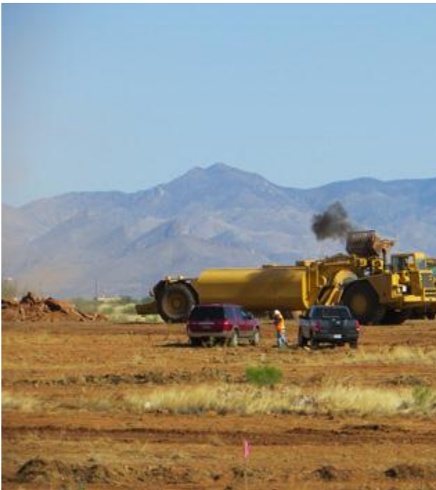
Bulldozers clearing the way for the solar array at the Fort Huachuca site.
