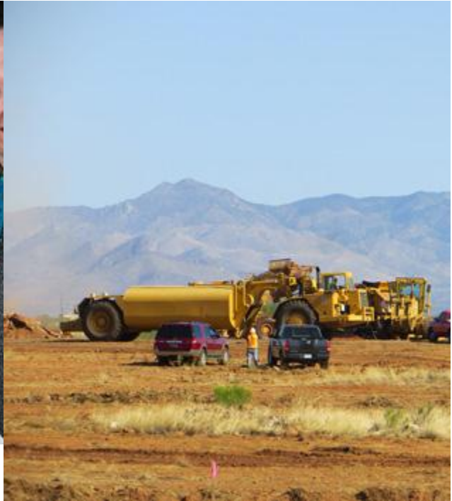
Bulldozers clearing the way for the solar array at the Fort Huachuca site.
