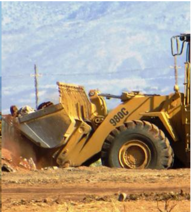
Bulldozers clearing the way for the solar array at the Fort Huachuca site.
